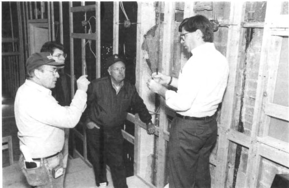
(Left to right) General contractor Bill Baldwin, DNALC Director David Micklos, CSHL Buildings and Grounds Director Jack Richards, and Centerbrook architect Jim Childress discuss renovation plans.
