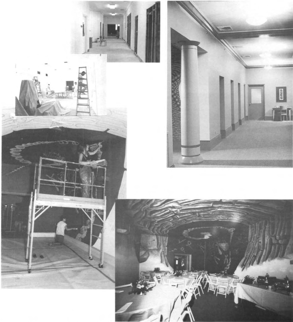
(Top) Refurbishment of front hall. (Bottom) Cellarium under construction, during painting and set for Corporate Advisory dinner.
